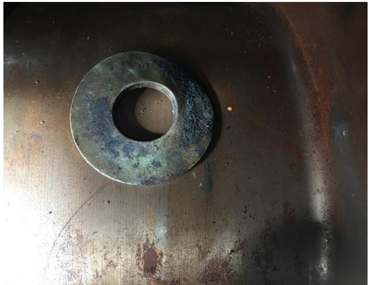
The equipment had cupped washers because the through-hole was so large that when it was bolted together, it mushroomed the washers.
