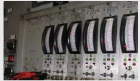
Fig. 1: Old BN rack where shaft vibration signals are easy to collect.
