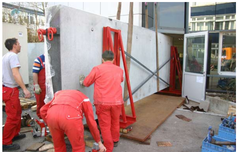
The delivery of the 12 m 2 12-tonne granite surface plate was no mean feat
