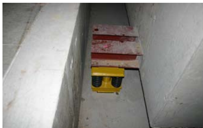
Seismographic measurements formed the basis of the interpretation and calculation of the dampers and the spring isolators
