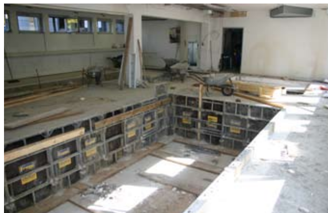
For a virtually vibration-free working surface, the concrete walls were mechanically separated from the building's foundation slab
