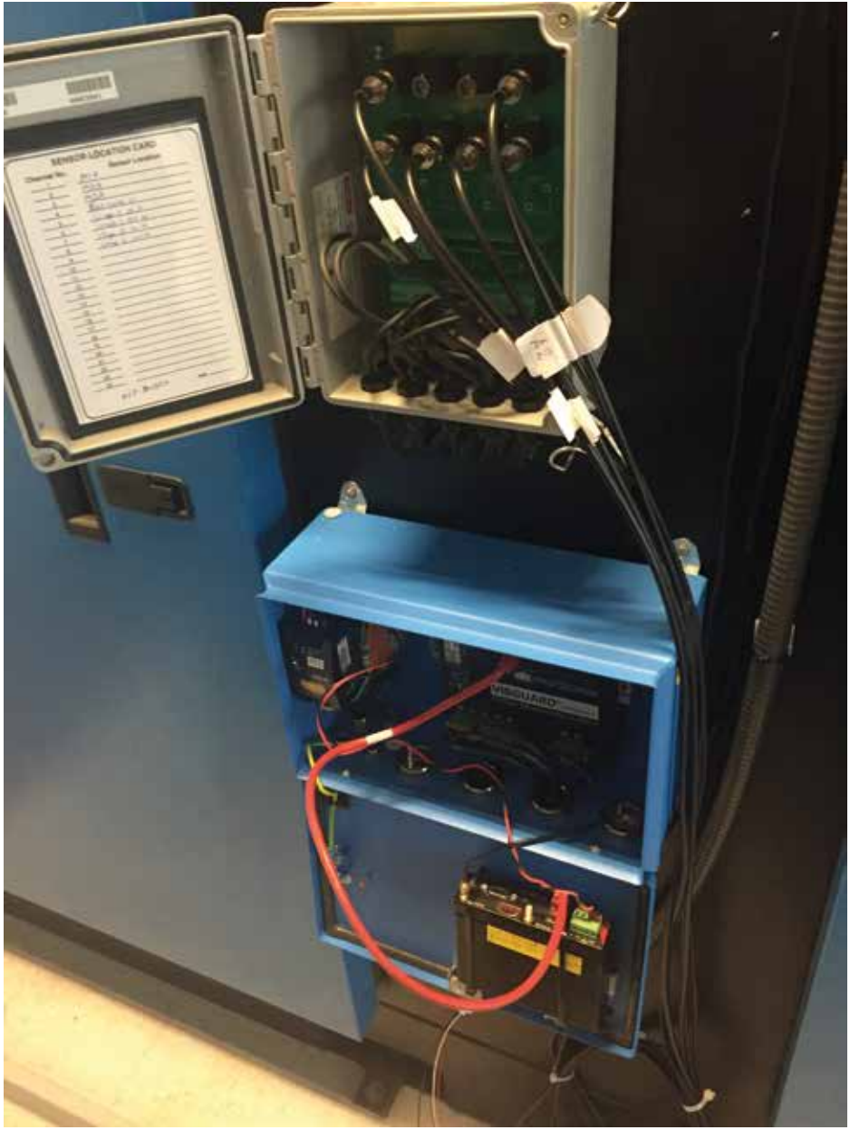
Figure 1: The junction box was already installed for connecting the PRUFTECHNIK handheld VIBXPERT® II which is currently used for route based monitoring of the compressor.
